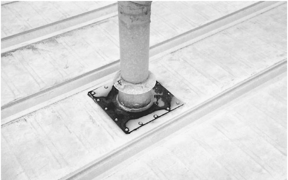
FIGURE 10.24 Damaged pipe boot flashing allows water to enter the building.
