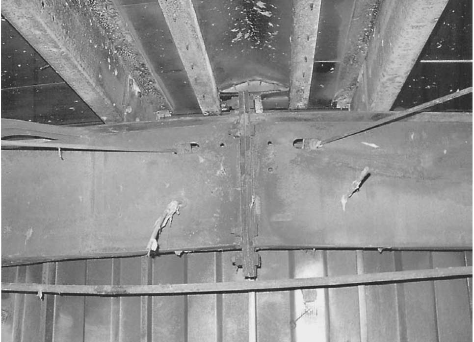
FIGURE 10.22 Effects of small fire on metal building system. The area at left is amplified in Fig. 10.23. Note also the method of rod attachment to frame. (Photo: Chabot Engineering.)
